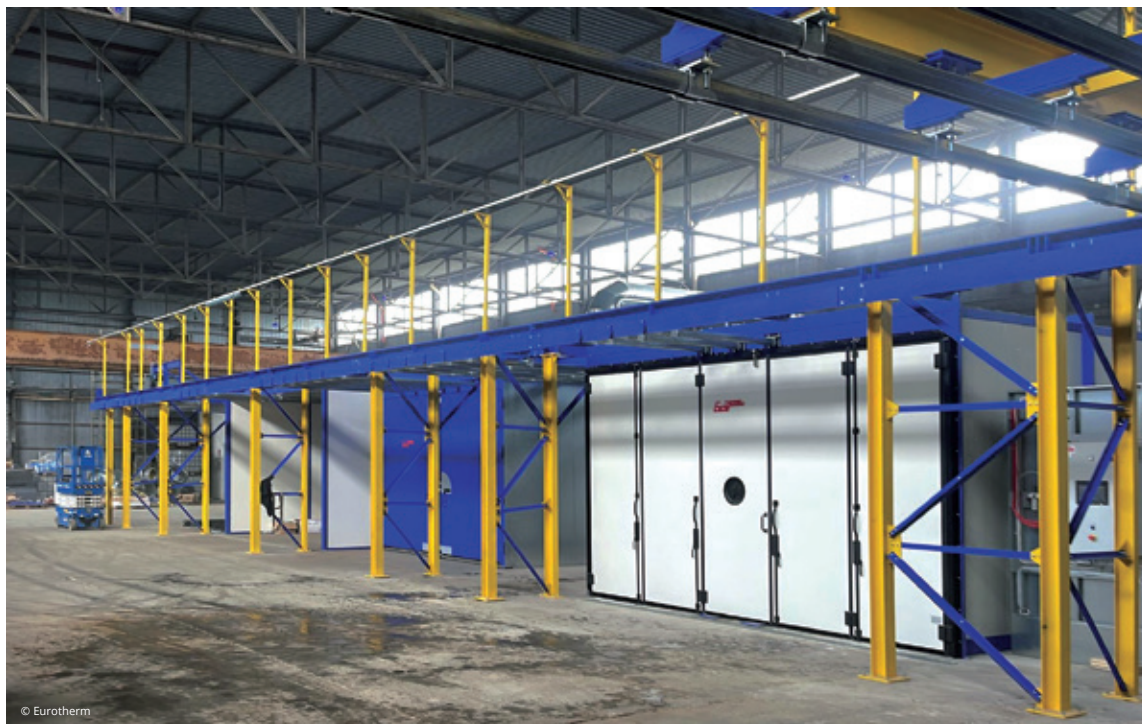
Overview of the Eurotherm shot blasting and powder coating plant.
