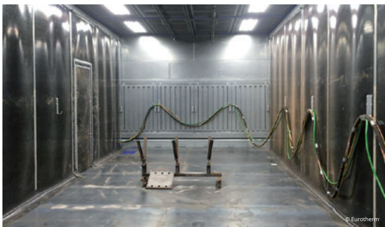
Inside the shot blasting booth, soundproofed to reduce the workplace noise level.
